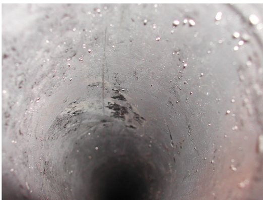
Fig. 4(c). Interior of the pipe (5 cm I.D.) after the third run at the highest oxygen concentration, showing significant oxidation and evidence of non-wetting.
